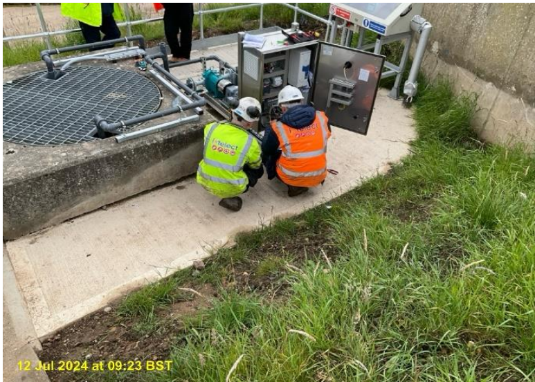
Dosing point being commissioned.
