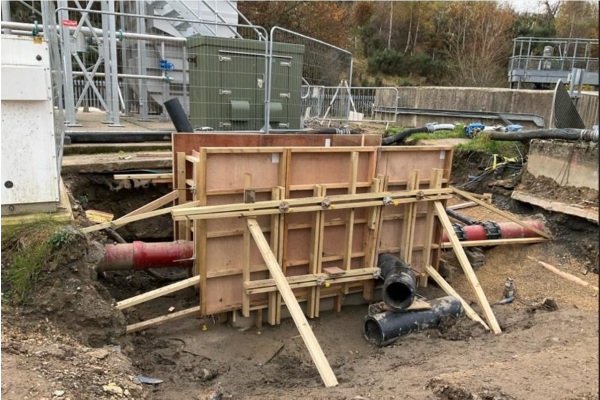
Flow Diversion Chamber
