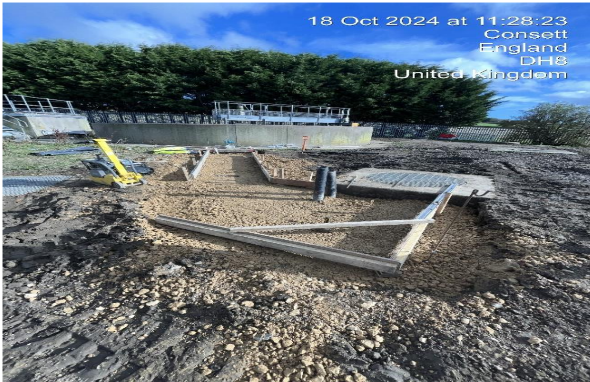
Caustic dosing POA slab
