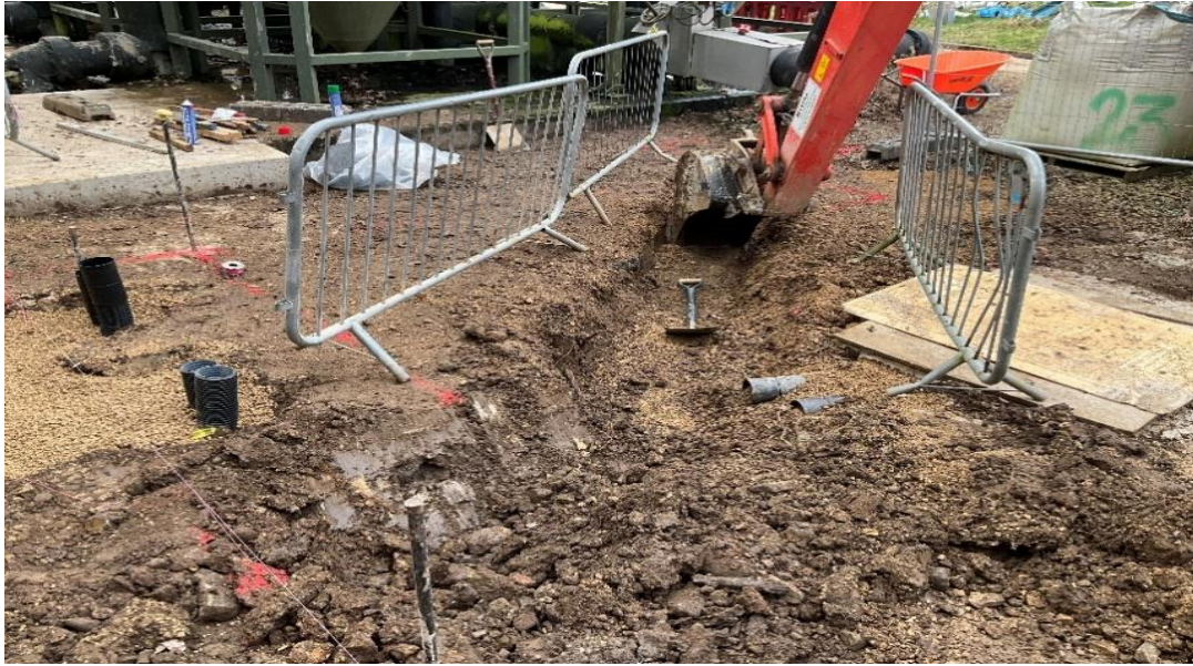
Ducts draw pit to kiosk
